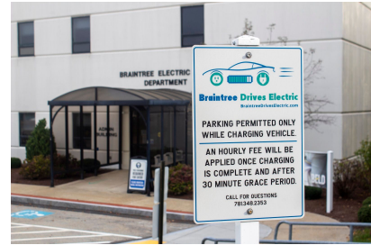
BELD's Charging Infrastructure
